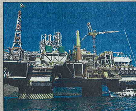
Step 5: Mating of the deck box with the lower hull successfully completed
